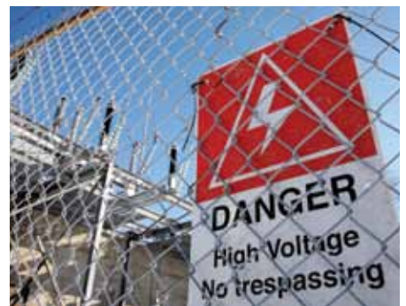
Never go into an electric substation for any reason. Electric substations contain high-voltage equipment, which can be deadly.
