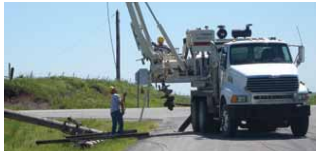
Caney Valley line crews worked diligently to restore members' power within just 48 hours.
