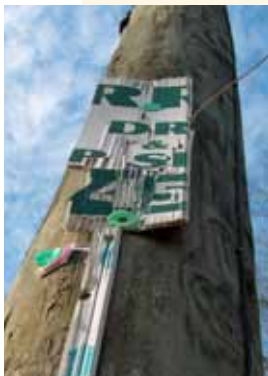
Staples, nails, and tacks used to hang signs pose dangers to Caney Valley Electric's linemen.
