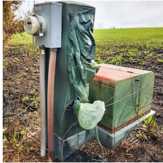
Before burning, check the property for electrical equipment — like this padmount transformer — and power poles to avoid damage and potential outages.
